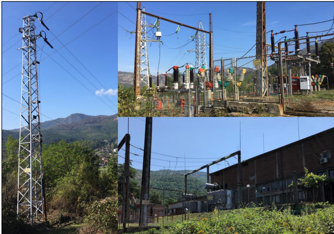
Figure 18-4: Pylon to support a 110 kV powerline and the Madzharovo substation Source: Velocity, 2020
